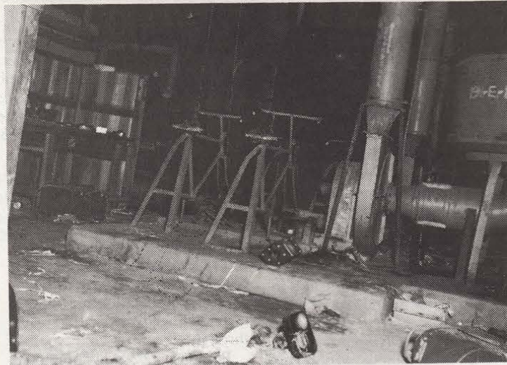
Air conditioning system consisting of six bicycle driven blowers.
